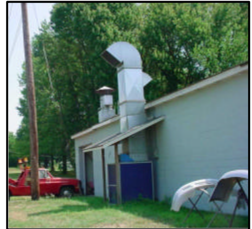
Vent design could cause odors to reach neighboring property
