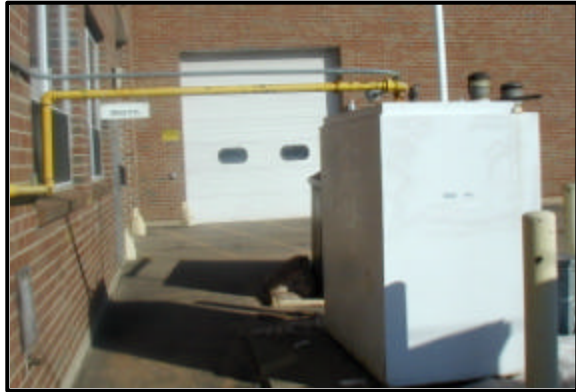
Double-walled above ground storage tank
